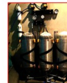
Compressed Air System
